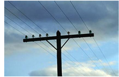
Long distance lines in classic copper technology
